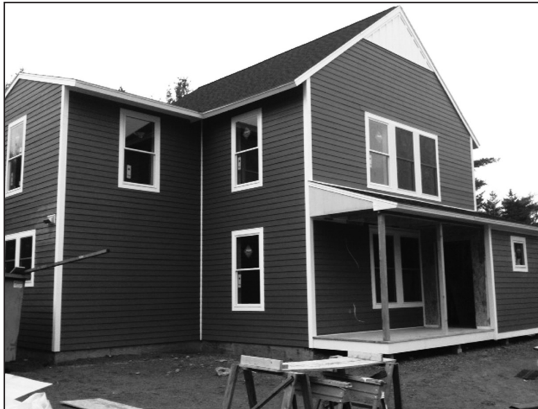
The sixth and final house in Phase 1 will be finished in January 2012 and will be home to an Acadia National Park employee, his wife and two young children.
